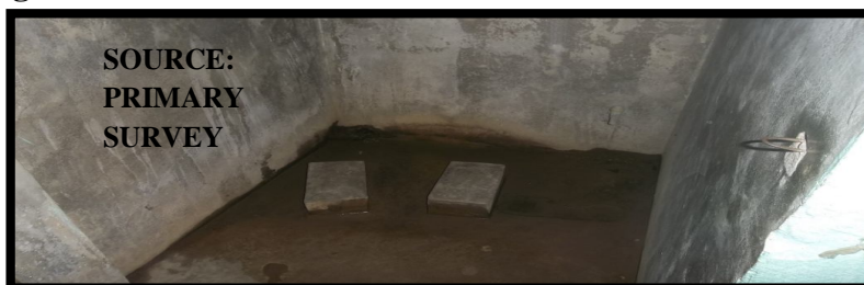
Fig 5: POOR TOILET CONDITION IN PUBLIC SCHOOL
